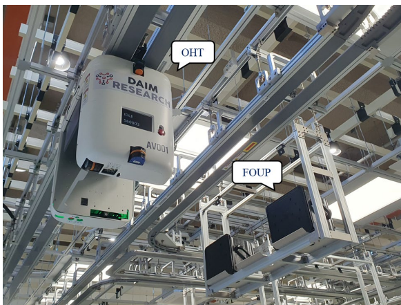
Figure 1. Components of an overhead transport system
